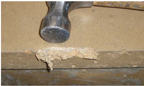
This “chip” was caused by repeatedly smacking the edge of the counter with a hammer. This is a good example for why we don't recommend you hammer on your countertop.
