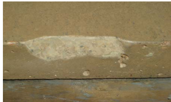
This same area is softened up by hand sanding it with 100 grit sandpaper. It should be re-sealed (not shown), to protect it and help it match the rest of the countertop.
